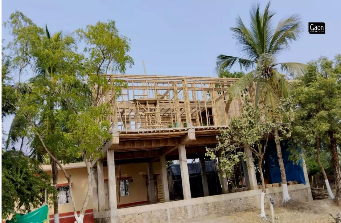
Figure 16: Construction of stilt house with concrete columns and foundation for better stability continued with the bamboo structure on top in Sundarbans
